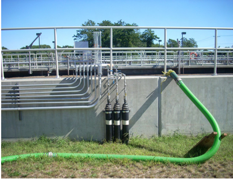
Fairfield methanol feed piping to secondary anoxic tanks
