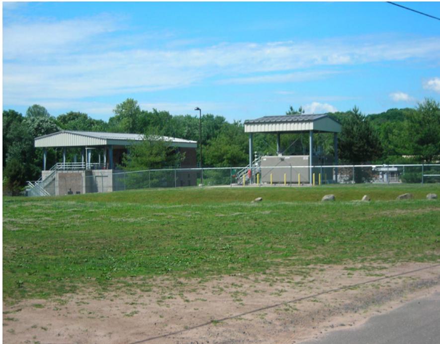
Figure1 - Cheshire denitrification filter and methanol storage facility
