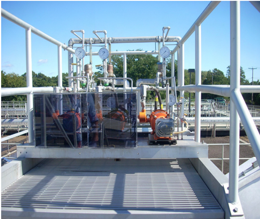
Fairfield Water Pollution Control facility explosion proof methanol pumps
