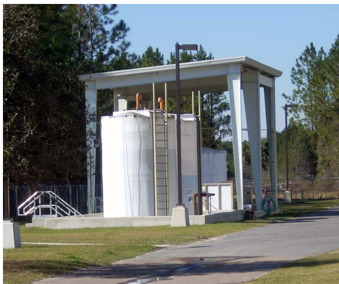
Supplemental Carbon Storage Tanks at Blacks Ford.
