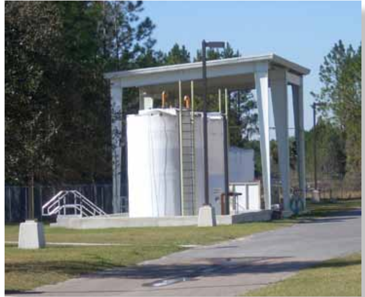
Supplemental Carbon Storage Tanks at Blacks Ford WRF
